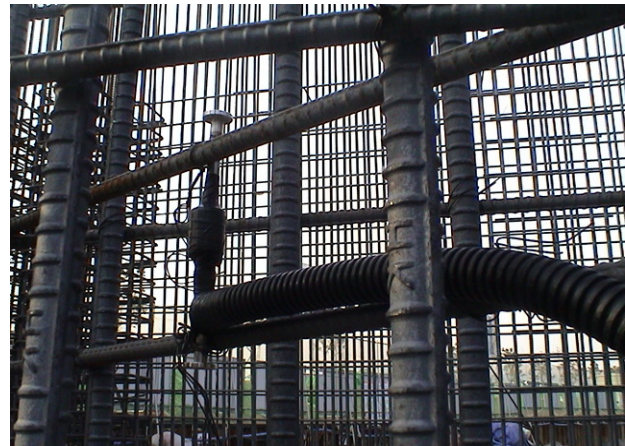
Fig.7. Vibrating wire strain gauge installed between rebars
