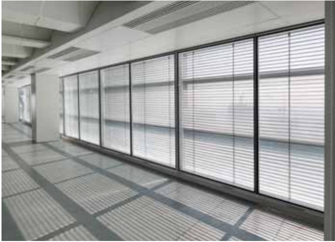
Figure 5. Motorized blinds/sunshade devices within the cavity.
