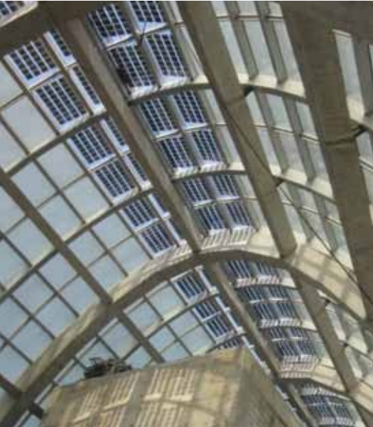
Figure 8. PV panels located on the roof.
