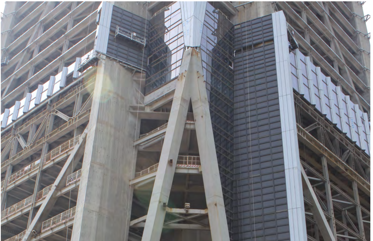
Figure 2.17. Installation of the façade (Source: Ping An) 图 2.17 独特外墙的安装 (来源: 平安)
