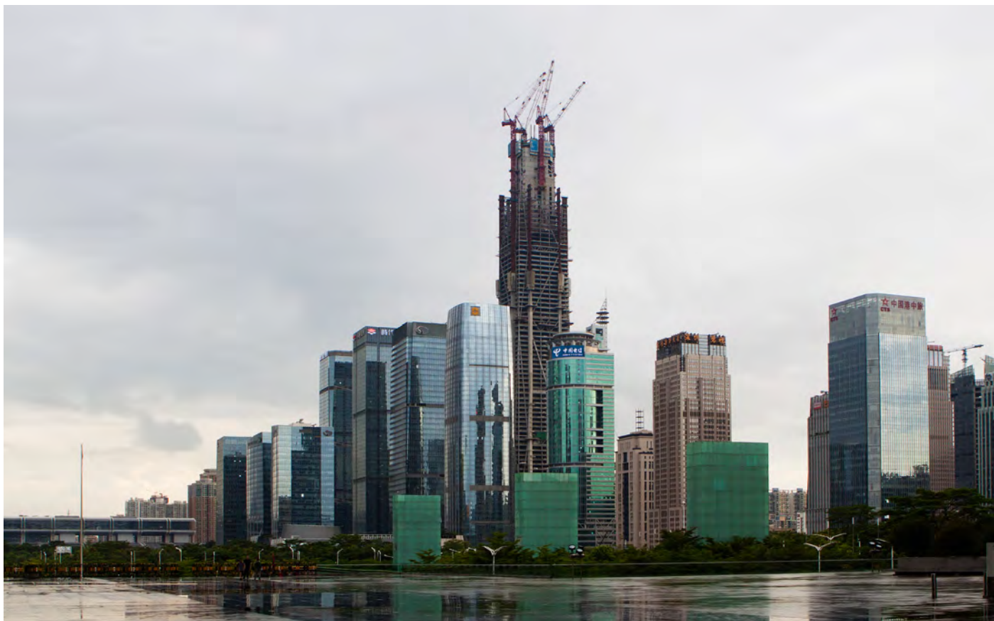
Figure 2.12. The Ping An Finance Center being constructed within the Shenzhen skyline (Source: Ping An) 图 2.12 深圳天际线中的平安金融中心的施工场景 (来源: 平安)
