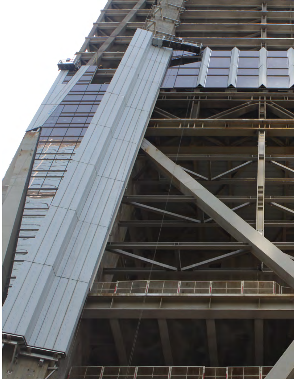
Figure 4.19. The stainless-steel façade being installed on the building. (Source: Ping An) 图4.19. 平安金融中心已安装不锈钢立面 (来源: 平安)
