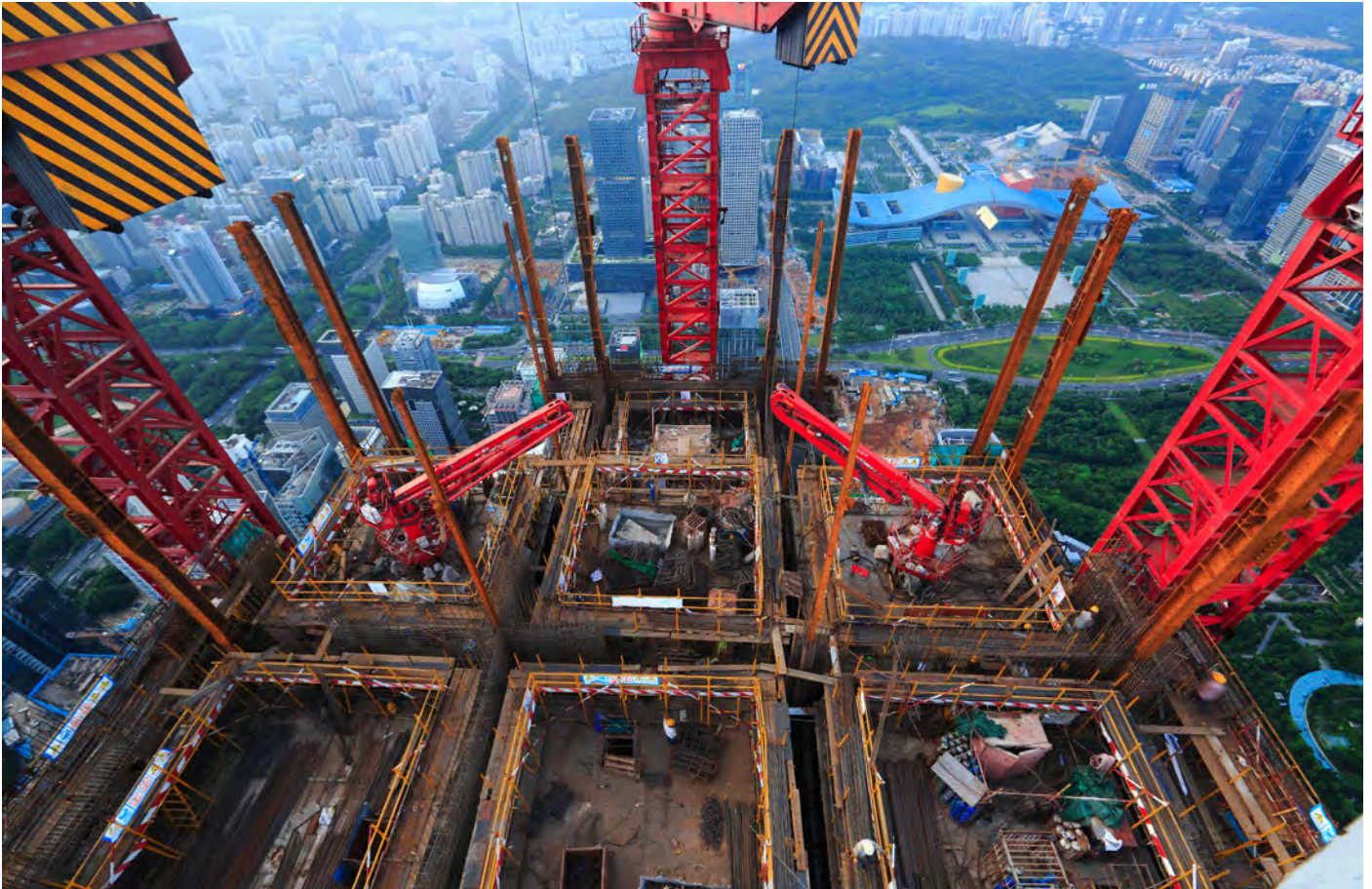
Figure 6.7. The goal of PAFC was to build one floor in four days, requiring appropriate tower cranes and climbing formwork (Source: Ping An) 图6.7. 平安金融中心的目标是一天建造四层楼，这需要合适的塔吊和爬模来实现 (来源: 平安)
