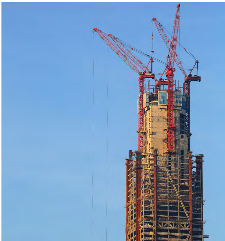
Figure 6.6. PAFc is a hybrid structural system composed of core walls, outrigger trusses and mega columns. (Source: Ping An)
