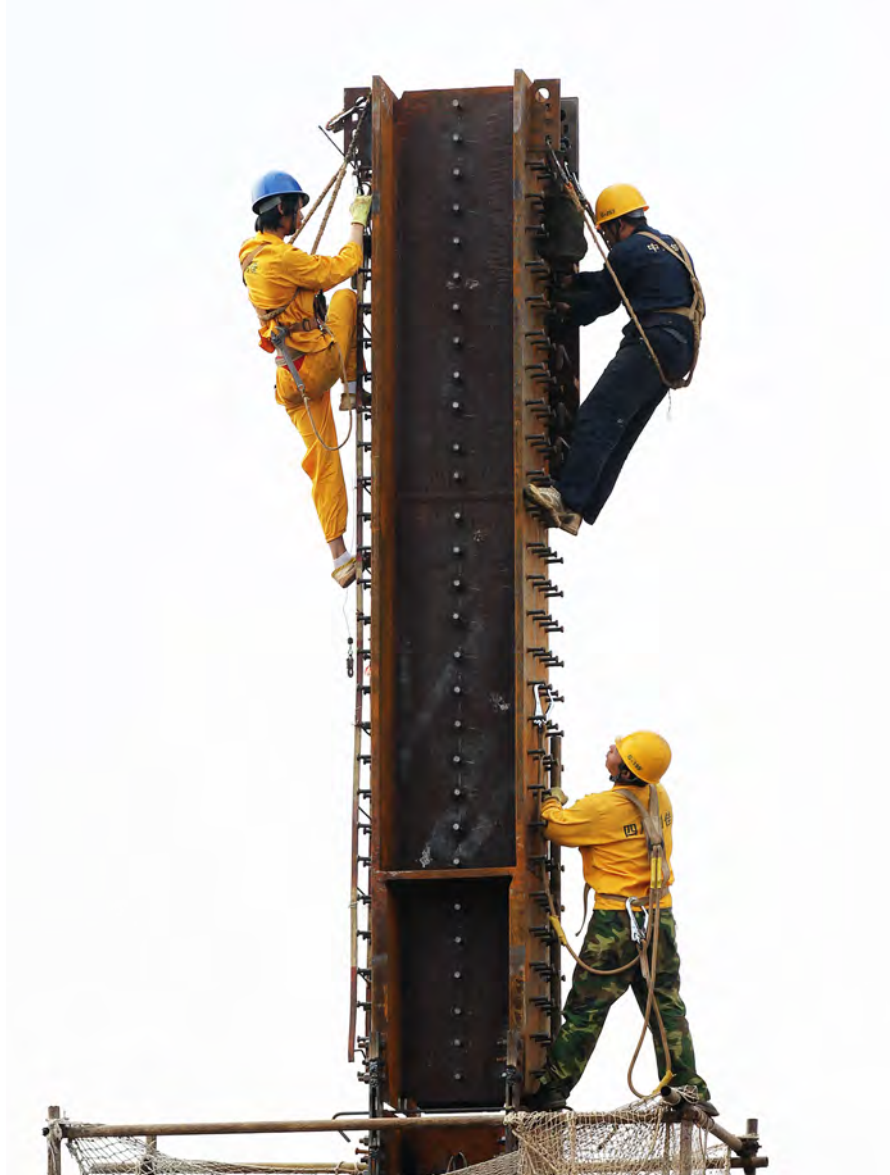
Figure 6.13. Fixing of mega columns on site. (Source: Ping An) 图6.13. 现场巨型柱子的安装 (来源: 平安)
