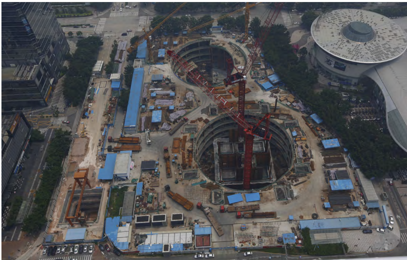
Figure 6.9. Completion of excavation at the site. (Source: Ping An) 图6.9. PAFC地基开挖完工 (来源: 平安)
