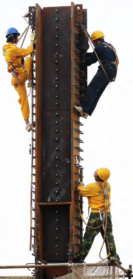
Figure 6.13. Fixing of mega columns on site. (Source: Ping An) 图6.13. 现场巨型柱子的安装 (来源: 平安)
