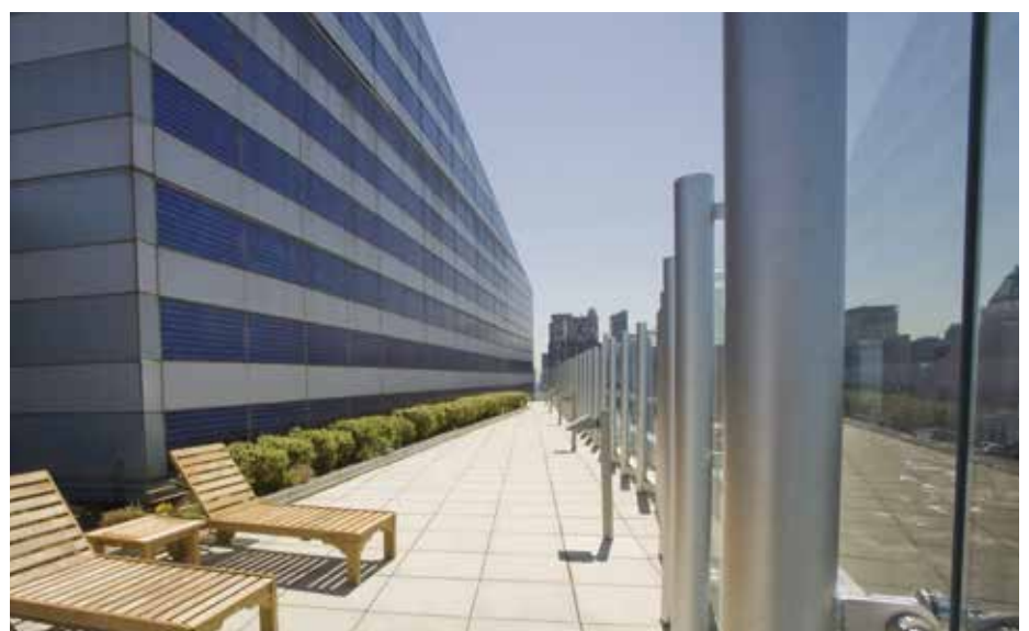
Figure 6. Roof installation of building-integrated photovoltaic solar panels at The Helena. (Source: The Durst Organization)
