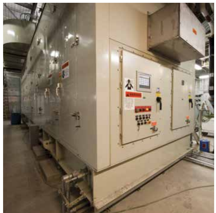
Figure 9. Installed cogeneration plant with onboard gas compressor. (Source: The Durst Organization)
