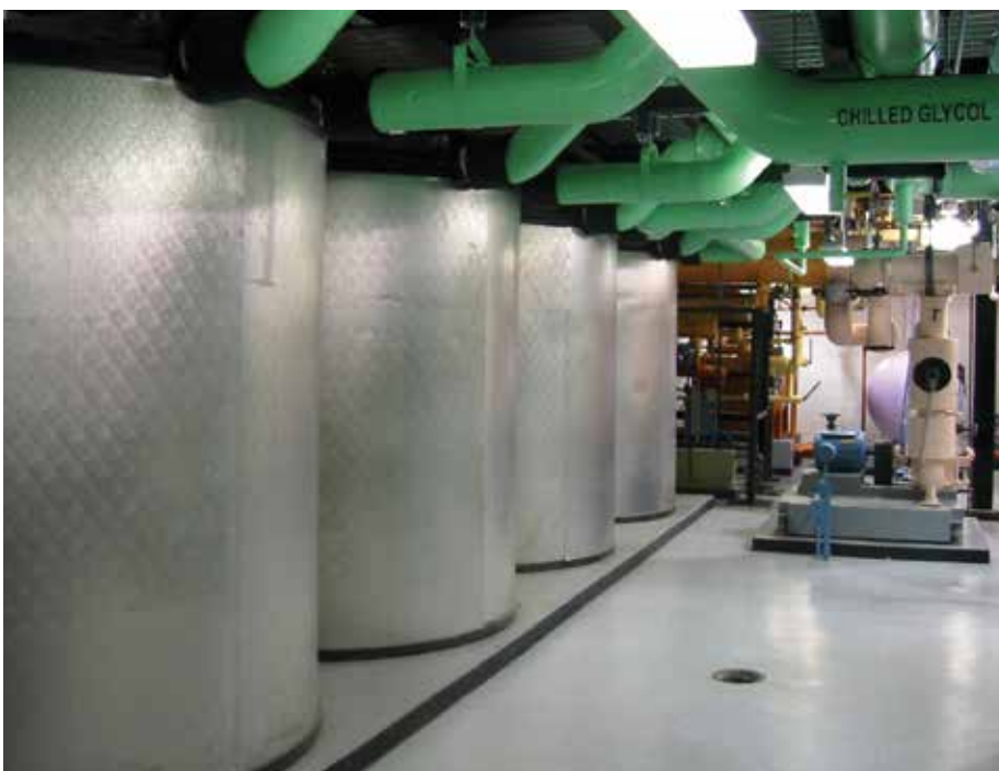
Figure 10. One Bryant Park's ice storage facilities allow the plant to run 24/7 while saving on energy costs. (Source: The Durst Organization)
