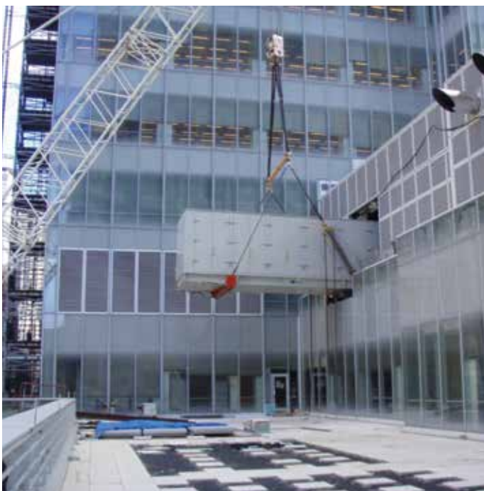
Figure 8. Installing the combined heat and power plant at One Bryant Park. (Source: The Durst Organization)
