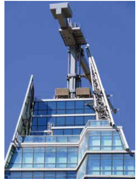
Figure 12. Damper Room (Source: Heerim Architects & Planners)
