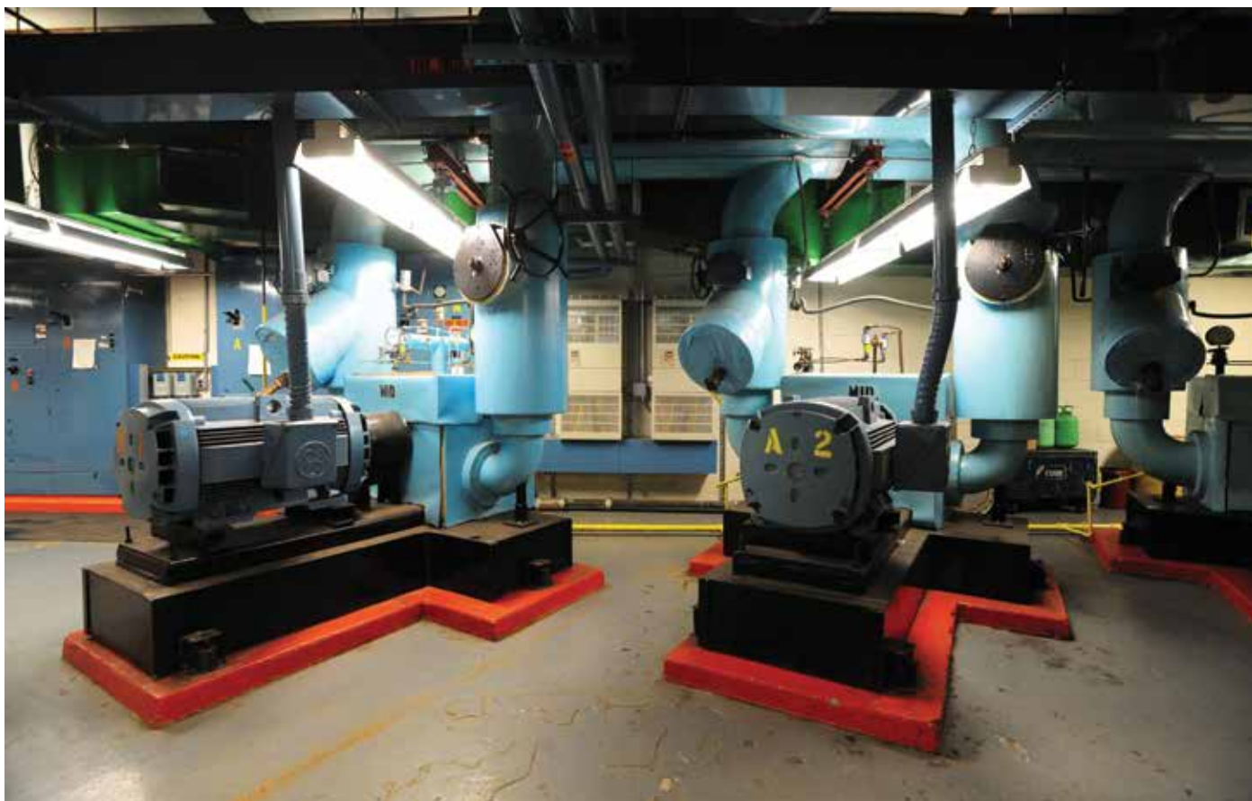
Figure 6. Chiller (Source: Empire State Realty Trust)
