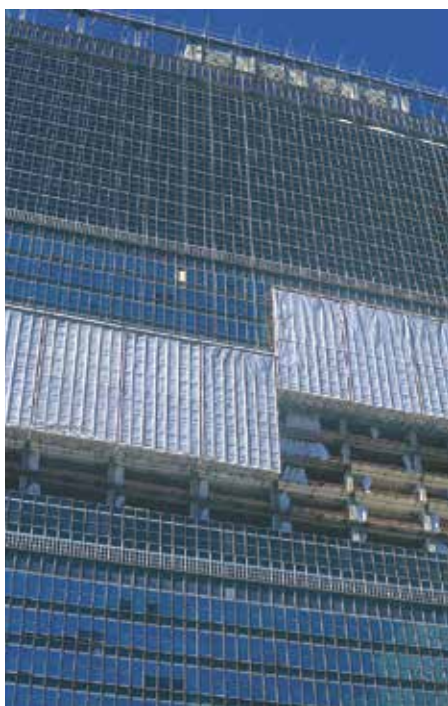
Figure 6. The new curtain wall being installed from the top of the Secretariat Building to the bottom, 2011 (Source: United Nations)
