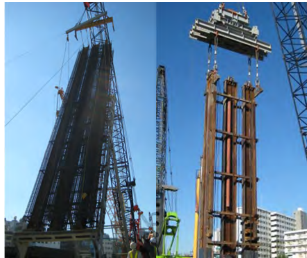
Figure 3.16. Device to stand the cage of steel frame (left). Figure 3.17. Device to have the cage inserted precisely (right).
