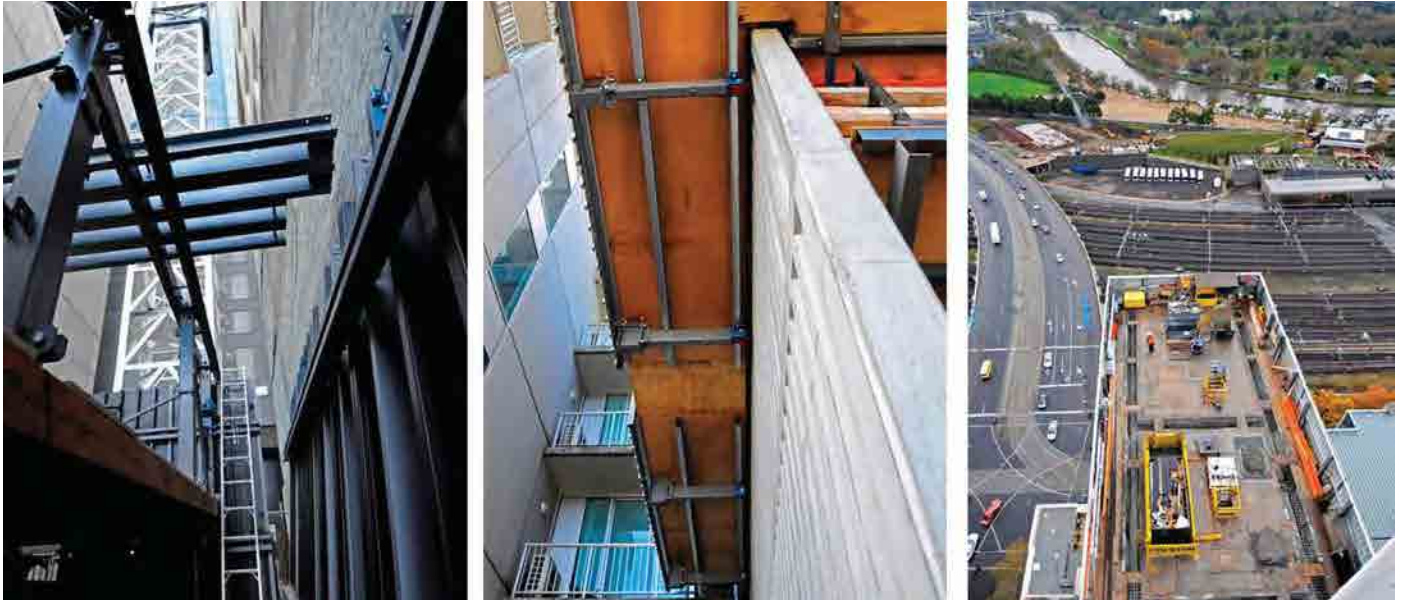
Figure 6. The structure and part of the envelope were rapidly built using a self-climbing jump-form system.
