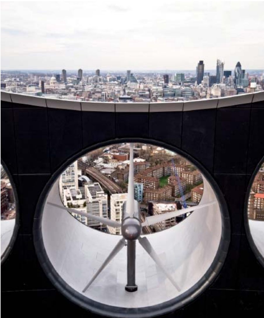
Figure 7. Strata SE1's five-bladed turbines © BFLS
