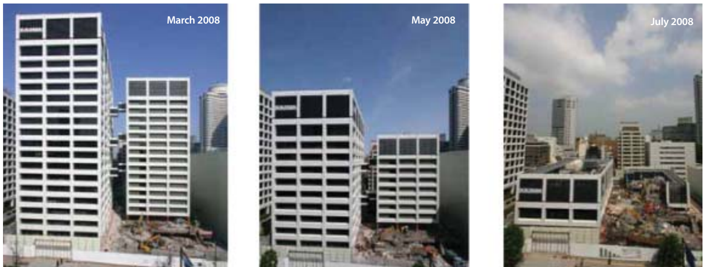
Figure 1. Kajima Cut & Take Down (C&TD) method used on Kajima's former headquarters in Tokyo © Kajima
