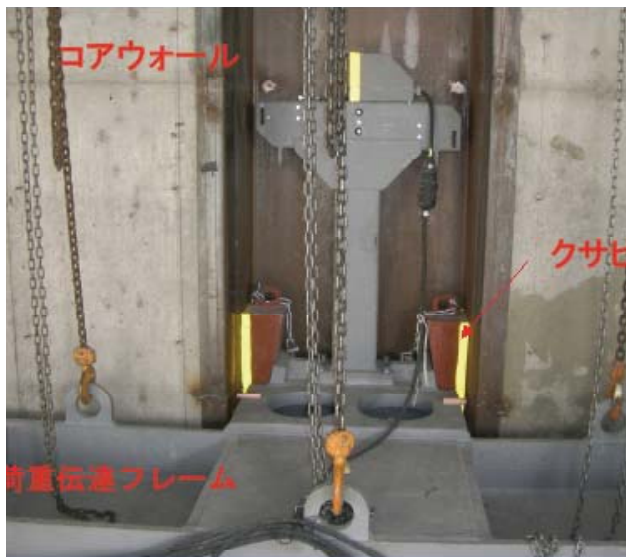
Figure 8. Wedge control device © Kajima
