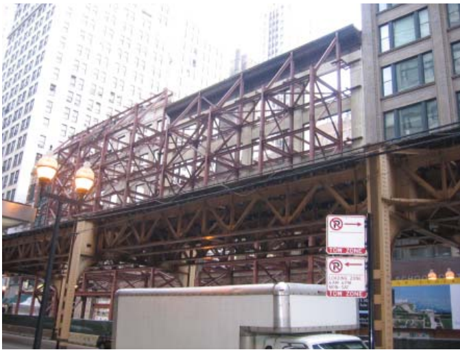
Figure 7. Temporary supports protecting historic façades, with “El” tracks in foreground © Walsh Construction
