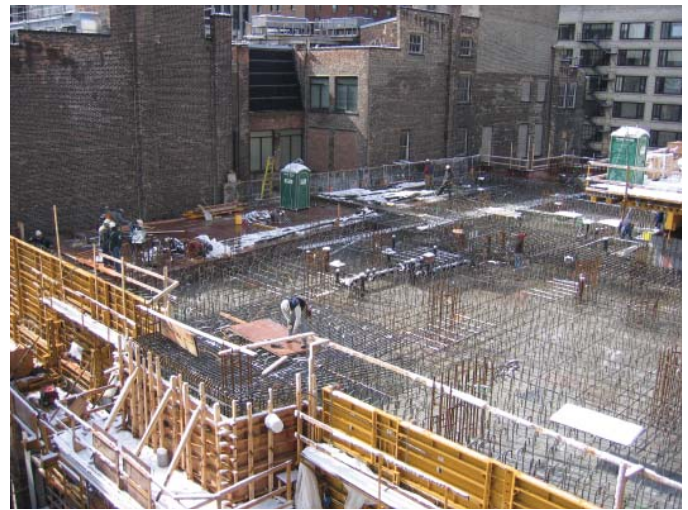
Figure 8. Third pour of mat slab with north wall of historic Sharp building to left of site © Walsh Construction
