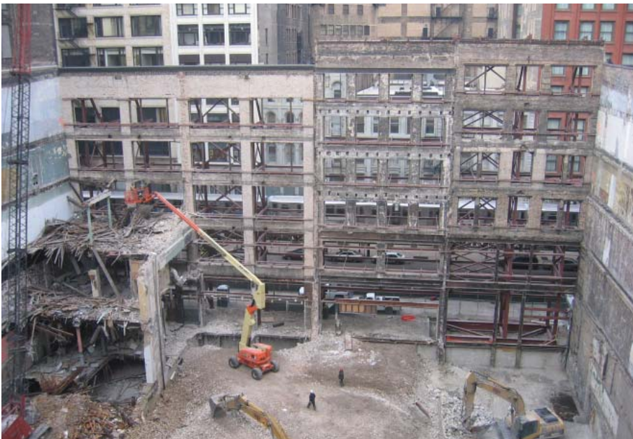
Figure 4. Demolition of vacant structures behind historic façades on Wabash Avenue © Walsh Construction
