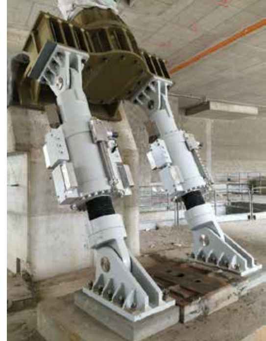
Figure 12. Viscous damper installed at the base of the steel struts in the Allianz Tower.
