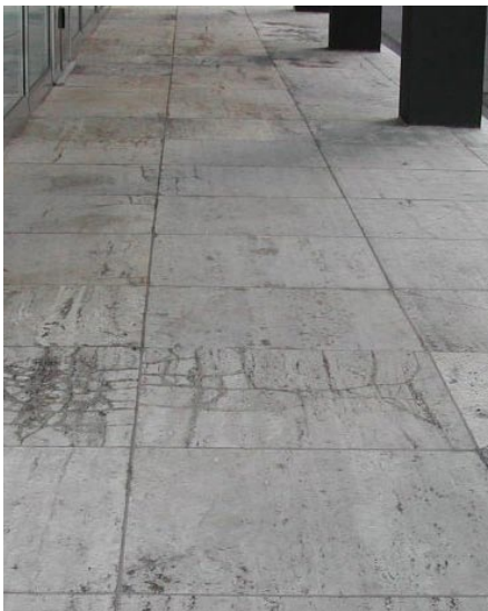
Figure 9. Travertine plaza deterioration. © Wiss, Janney, Elstner, Associates
