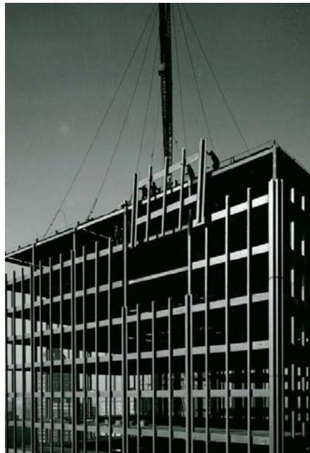
Figure 3. Prefabricated façade panels lifted and welded into place ca. 1951. © Hedrich Blessing Collection, Chicago History Museum
