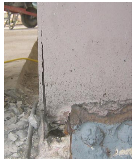
Figure 8. Weld split at steel faced column due to corrosion. © Krueck & Sexton
