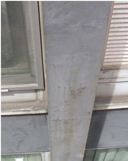
Figure 5. Steel corrosion and paint deterioration. © Wiss, Janney, Elstner, Associates
