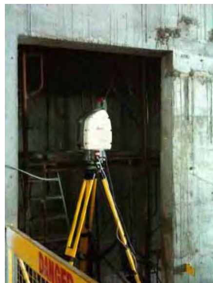
Figure 4. 3D laser scanning for the lift core (Source: Daewoo E&C) 图4. 用3D激光扫描仪扫描电梯井道 (出自: 韩国大宇工程建设公司)
