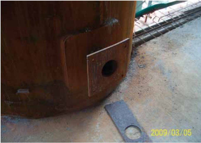
Figure 5. Connecting end interface design with steel tube column (source: Yang Yaohui Gao Junfeng & Wang Jing) 图5. 与钢管柱连接端顶升接口 (出自: 杨耀辉)
