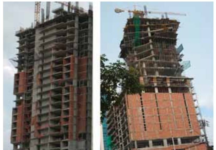
Figure 4. Brick Infill Cladding with No Movement Joints (source: Magnusson Klemencic Associates)
