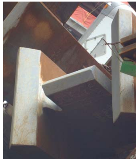
Figure 2. Column splicing Jumbo beveling (Source: ArcelorMittal) 图2. 巨型斜角拼接而成的柱子 (出自: 安赛乐米塔尔)
