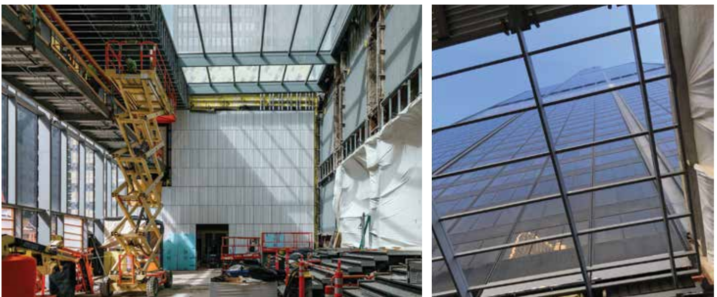
Figure 4. A view of the Wacker Lobby under construction, with white terra cotta panels (left) and a skylight view of the tower (right). © Gensler
