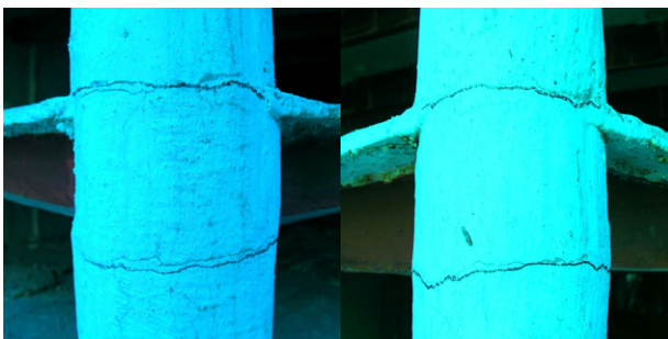
Fig. 4. the Typical Cracks on the SRC Columns
