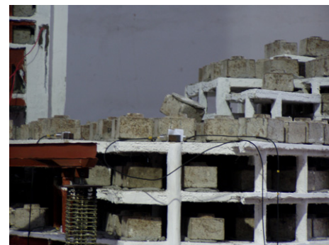
Fig. 8. Collapse of Roof Frame of the Podium
