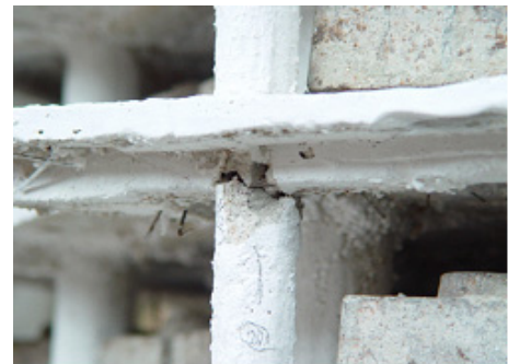
Fig. 7. Cracks of Podium Frame
