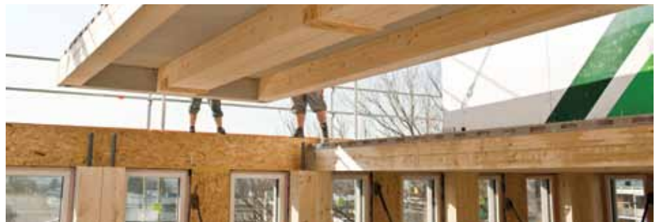
Figure 1. Timber-Concrete-Composite (TCC) slab. After all the walls are installed, the floor slabs, which were fabricated with a hole in each corner, slide over the pins in the glulam posts. © CREE
