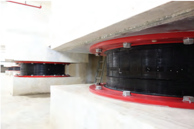
Figure 8. High damping rubber bearings in Gudang Garam Office Tower (Source: Davy Sukamta)
