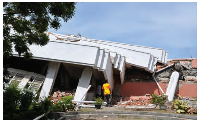
Figure 1. Total collapse of building in Padang during the S.Sumatra M7.5 EQ in 2009 (Source: Davy Sukamta)
