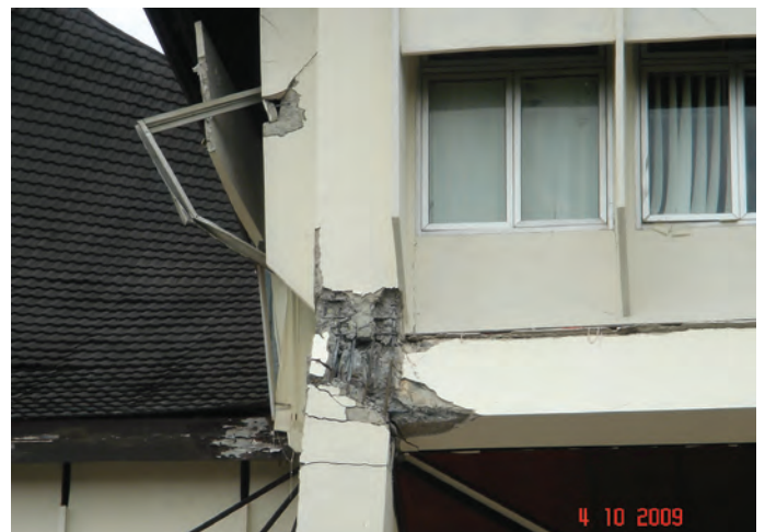
Figure 2. Beam-column joint failure in RC Beam in Padang during the S.Sumatra M7.5 EQ in 2009 (Source: Davy Sukamta)
