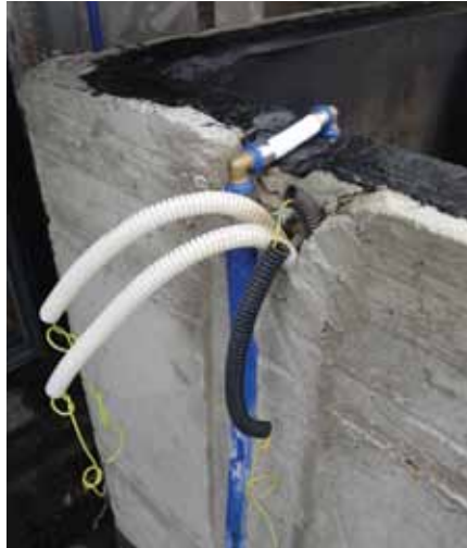
Figure 11. Plant containers' drainage system.
