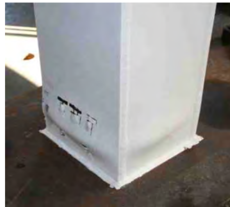
Figure 12. Confirmation of failure mode.
