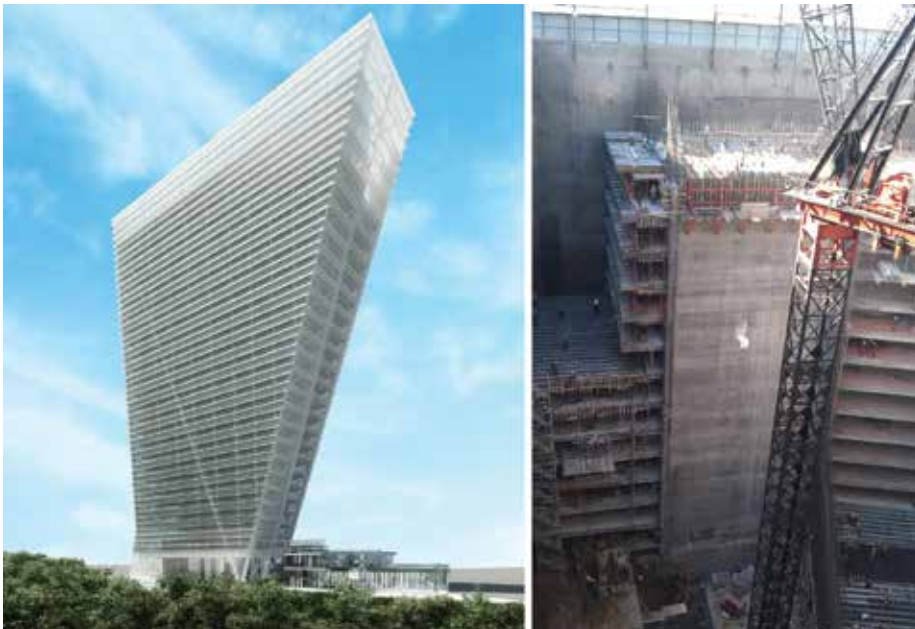
Figure 2. (Left) the impressive 75m cantilever at 24 Pedregal protects the existing Vladimir Kaspe Building. (Right) Pedregal's 16 story basement – the deepest in Latin America (Source: Arup)
