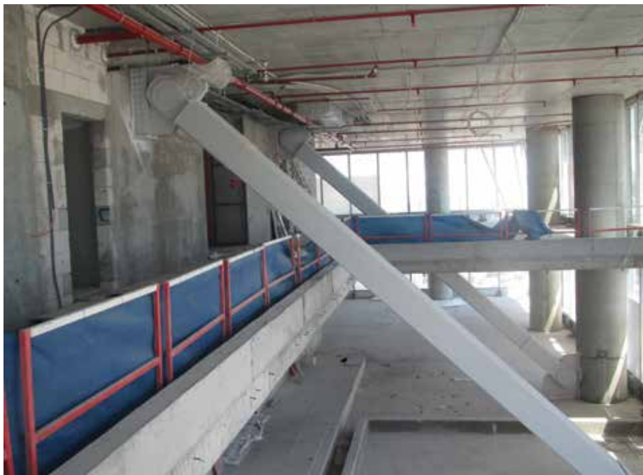
Figure 15. Allianz Tower. Buckling restrained braces—located in the middle of the tower. (Source: FXFWOLE)
