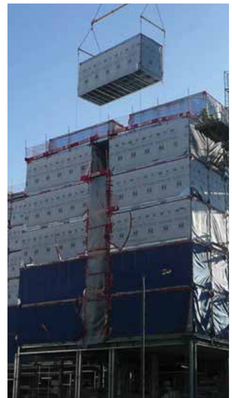
Figure 1. Modular technology like PPVC is a viable tall building solution (Source: Ramboll Group)
