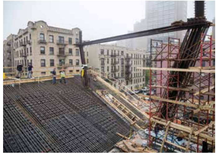
Figure 14. Combination of state-of-the-art materials and technology: void formers, high strength rebar, high strength concrete, and structural steel embedded in columns form the Auditorium structure at the base of the Cascade (Source: Matthew Melrose)
