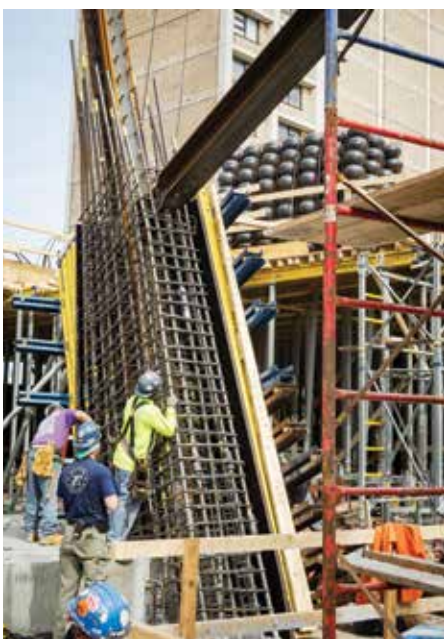
Figure 13. Special attention was paid by the Construction team to unique structural details when building the architecturally exposed columns in the Cascade (Source: Matthew Melrose)
