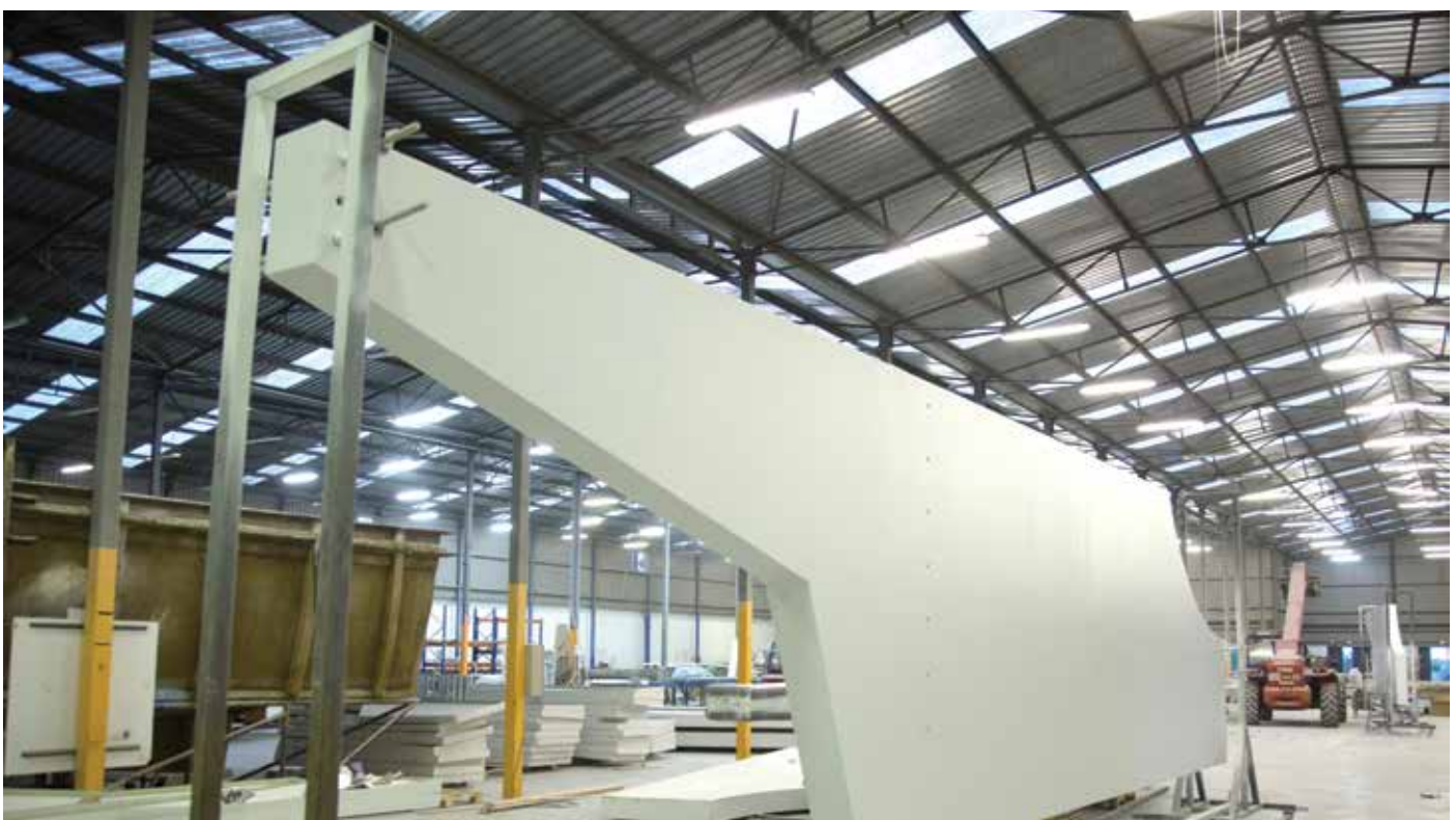
Figure 13. A fin after painting, during its curing process (Source: ENvolventes ARquitectonicas - ENAR)
