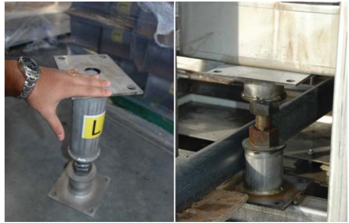
Figure 9. The pool's adjustable steel jacks
