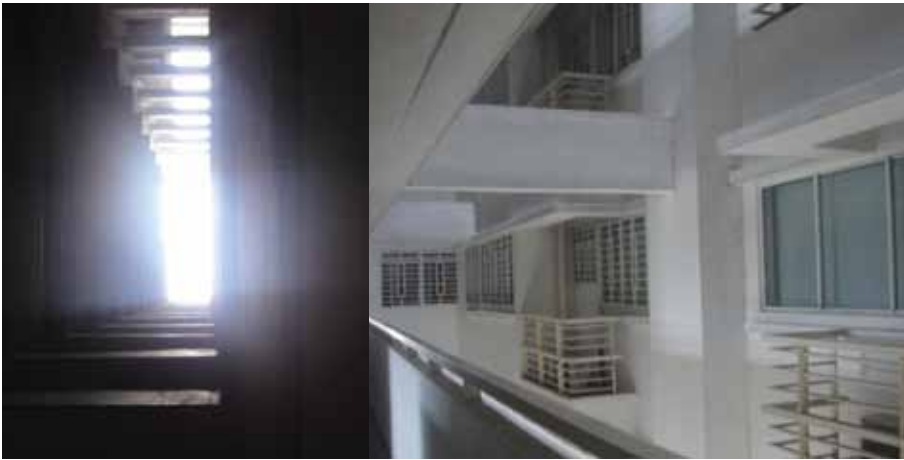
Figure 8. Shallow depth of floor voids
