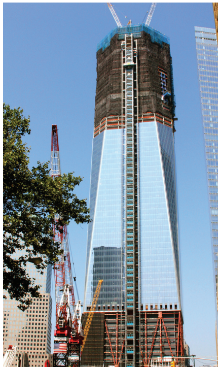
One World Trade Center, New York will be the newest US supertall when completed in 2013 © CTBUH
