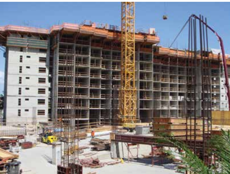
Figure 5. Affordable tunnel form tower under construction uses poured concrete walls, which are erected quickly and create a durable unit. © Steven Baldrige
