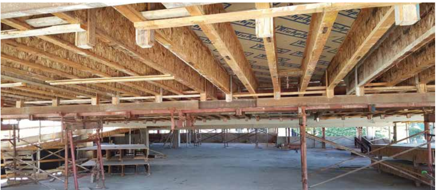
Figure 7. Garage slab form panels can also be moved relatively easily up parking structure ramps. © Steven Baldrige
