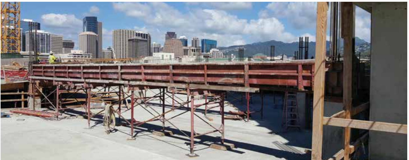
Figure 6. Garage beam steel forms can be moved easily, cutting down on costly crane operations. © Steven Baldrige
