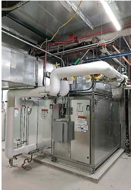
Figure 6. View of a typical floor-by-floor AHU. © Environmental Systems Design, Inc.
