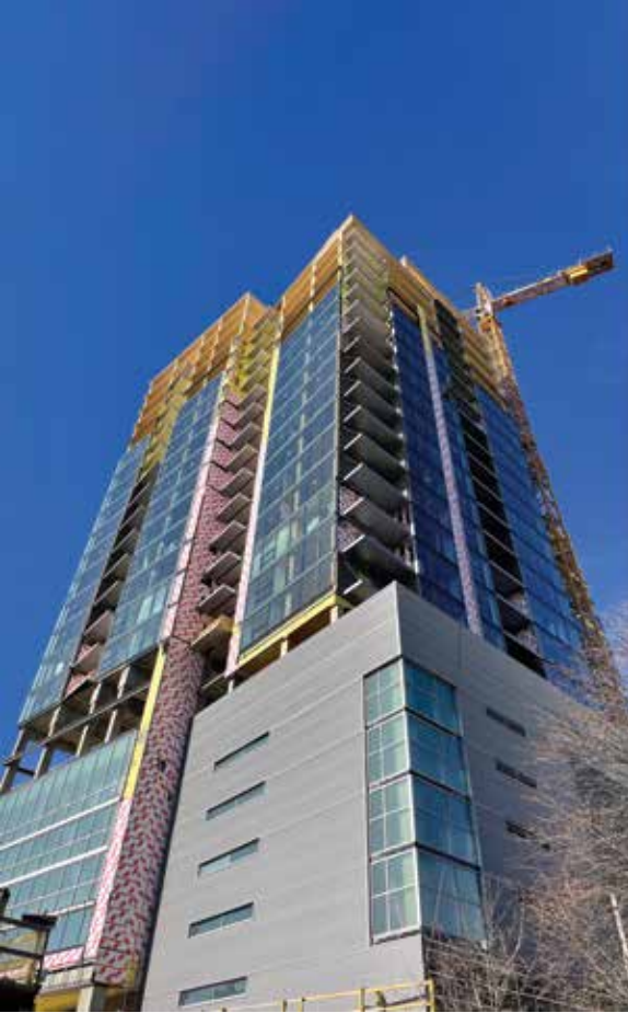
Figure 2. Ascent, Milwaukee, USA, 86.5 meters and 25 floors, is expected to become the world's new tallest timber building when it completes in August 2022. © C. D. Smith Construction
