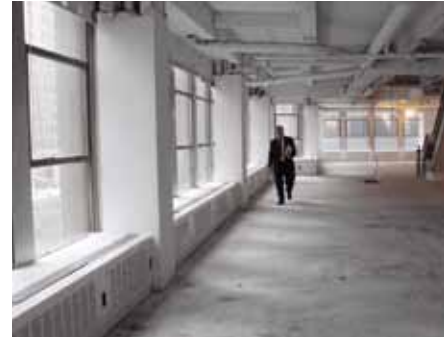
Figure 3. Existing perimeter induction units used to distribute air from the central fan rooms.
